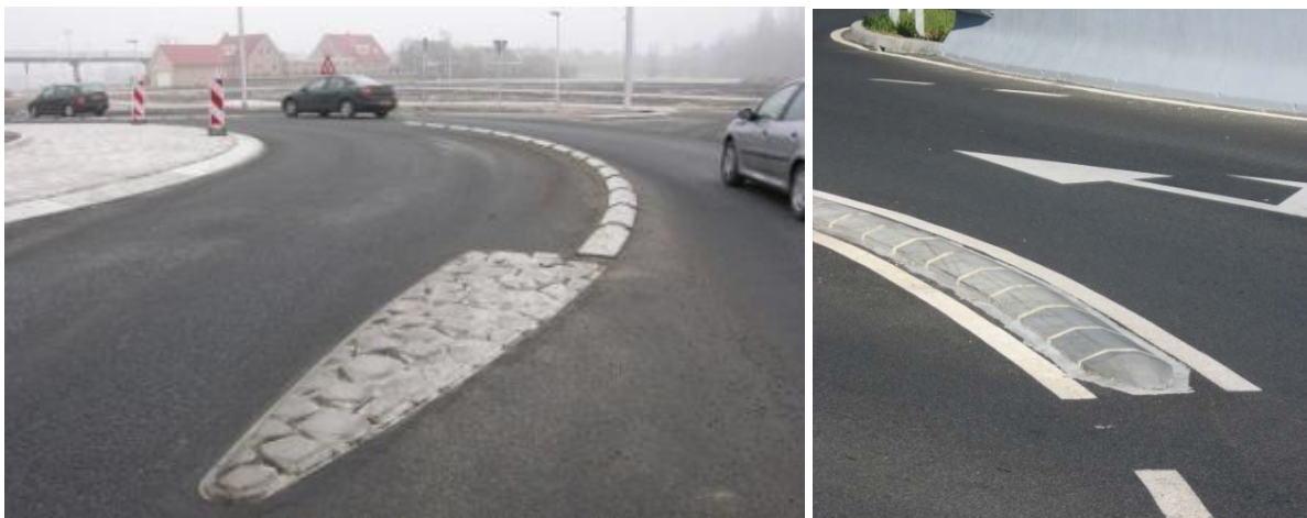
Figure 21. Different construction of starting area of the dividing element: in the Netherland (left) and in Slovenia (right)
